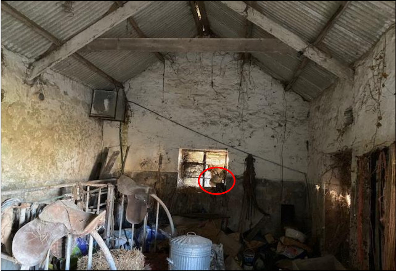
Figure 4. Internal view of the barn with the broken window on the northern gable end highlighted.
