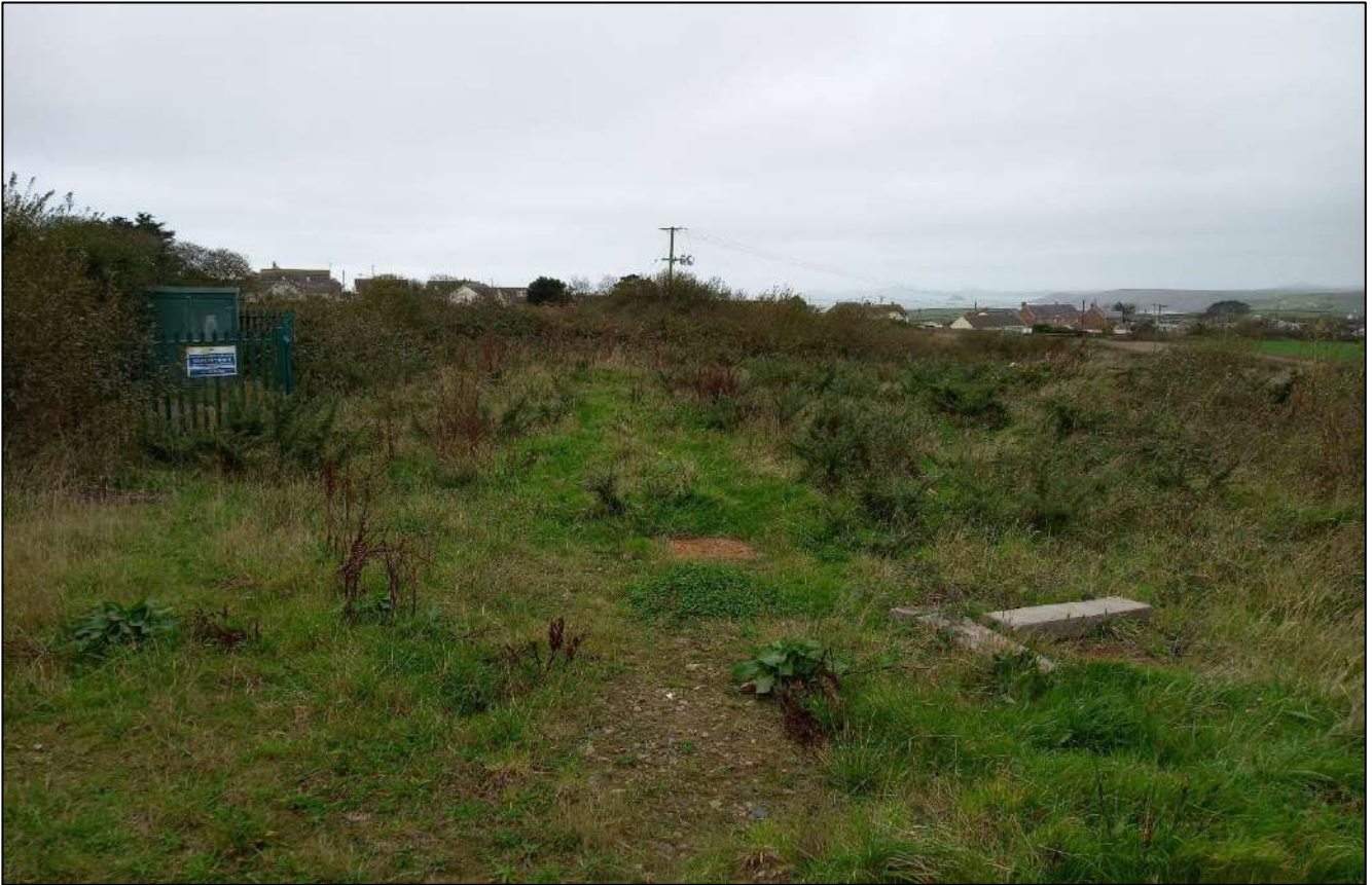
Plate 19. Foul water pumping station for Maes Ffynnon in south of the north-east field of the PDA, looking south-west.
